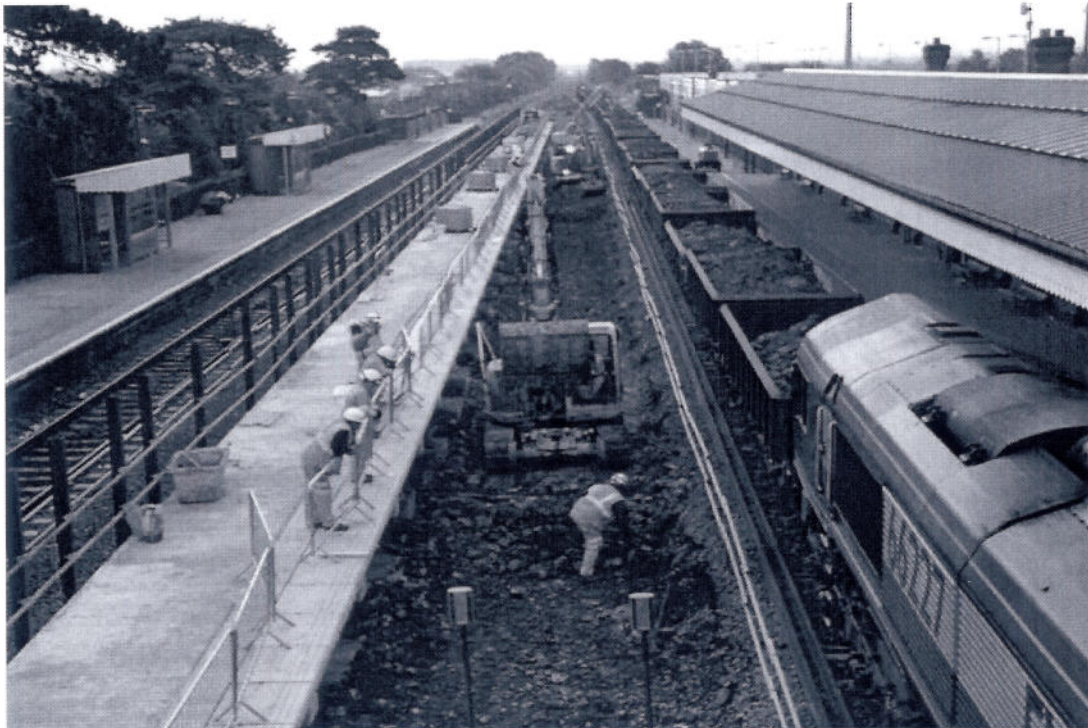
The picture shows Chiltern Railways delivering the new platform at BicesterNorth Station as part of Evergreen 3, phase 1.
